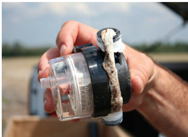
Figure 15. Filamentous sulfur slime completely clogging a small water meter.
