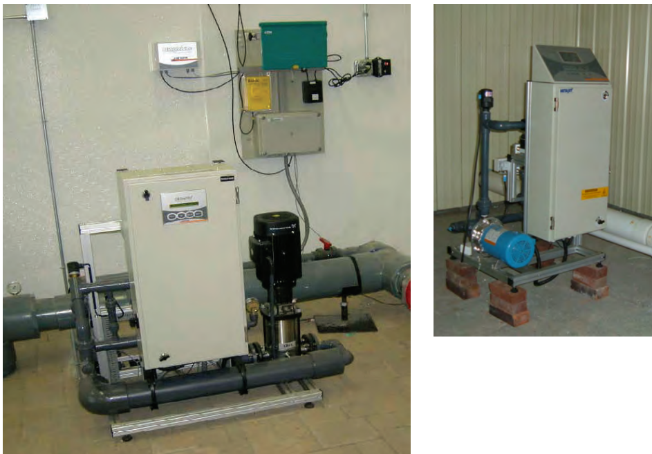
Figure 4. Examples of a Netafim fertilizer injection and irrigation control system.
