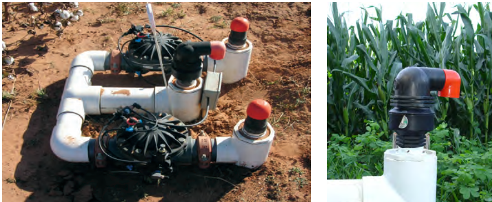
Figure 3. Examples of a field installation of Pressure Regulating Valves and Air/Vacuum Relief Air Vents.
